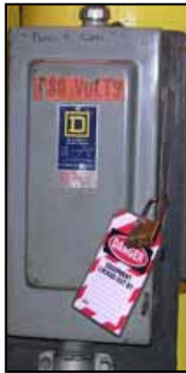
Figure 1: Lockout/Tagout on the Power Source Panel
